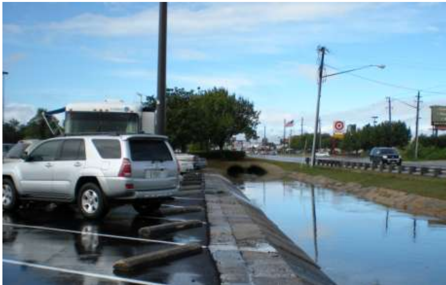
Figure 2 After a recent rain, a stormwater ditch and culverts at the Panama City Mall. Bay County, Florida.
