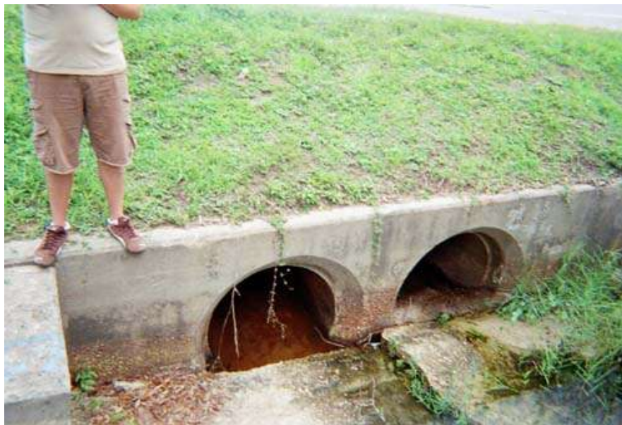
Figure 6 FSU volunteer intern Matt Beard prepares to record data at stormwater outfall pipes located in the City of Parker. Eastern Bay County, Florida.
