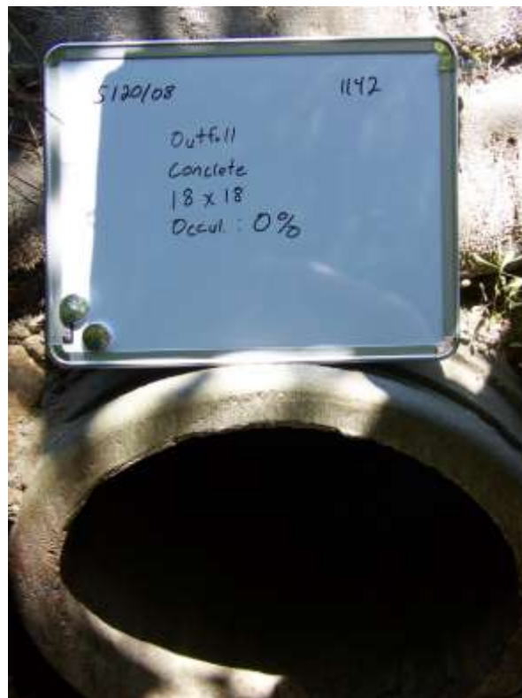
Figure 8 Outfall pipe and corresponding data, located in Southport. Northern Bay County, Florida
